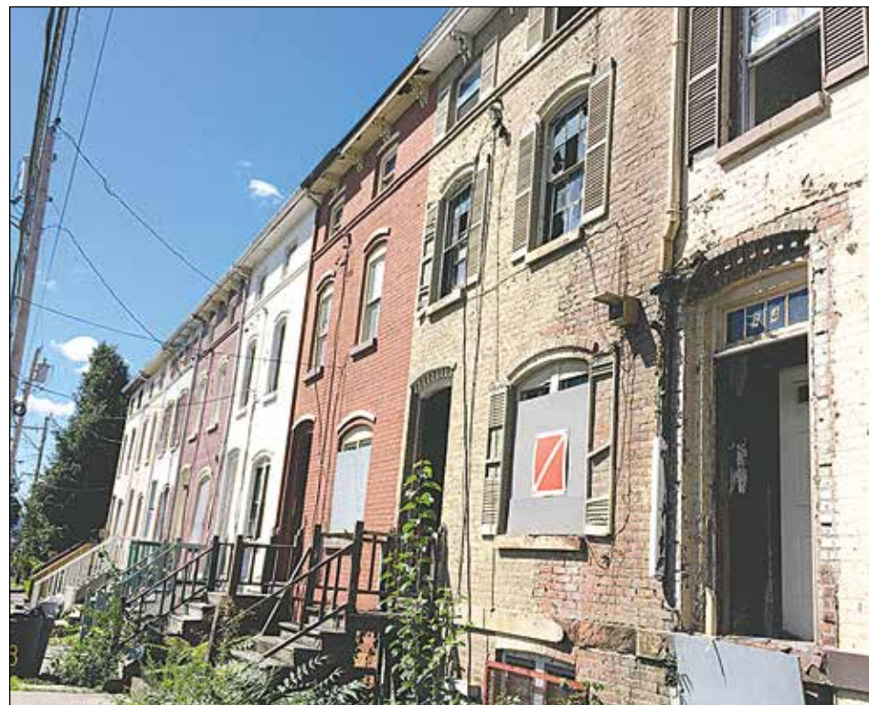
Red signs alert city workers to enter buildings at their own risk on Lander Street.
