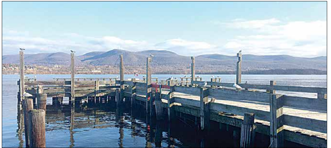
The ailing Newburgh Landing Pier.
