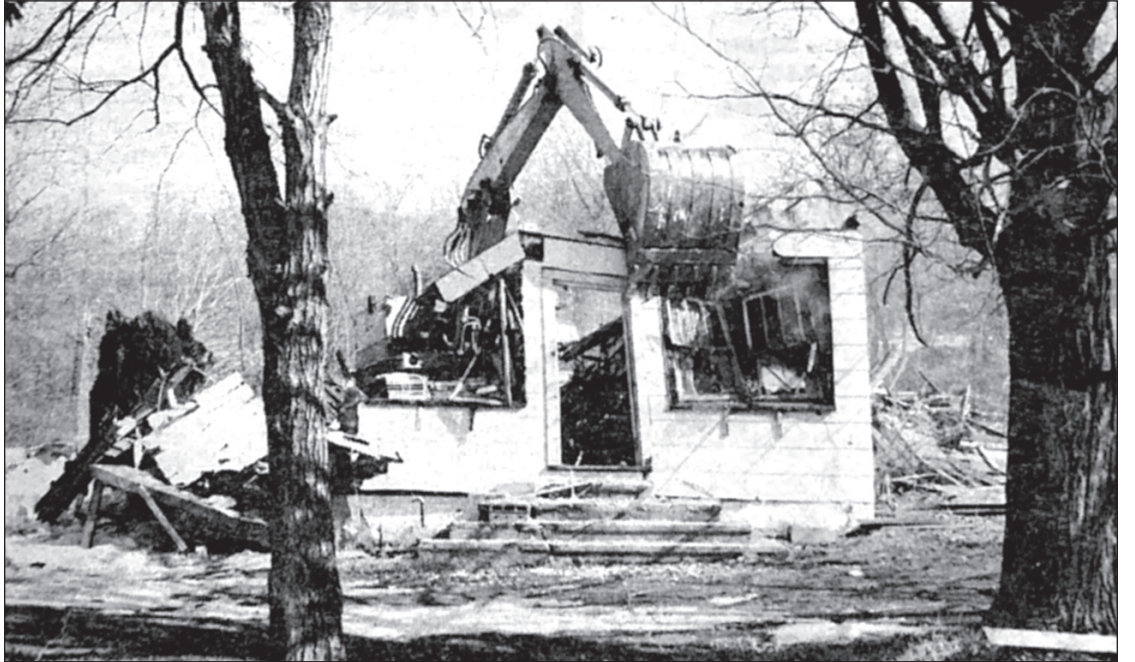
March 1987: A large backhoe puts the finishing touches on an abandoned building at the intersection of Routes 17K and 208. The building, once a State Police substation, came down to make room for the Walden Savings Bank Corporate Headquarters.
