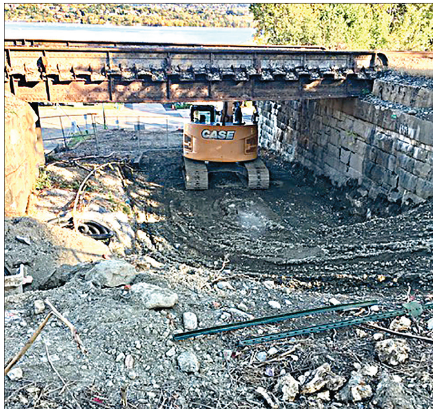
An excavator reveals Fifth Street where it runs between Water and Front.
