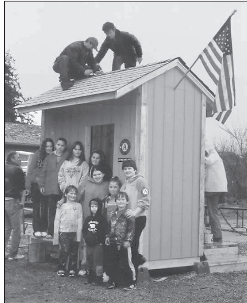
AmeriCorps-led volunteers rebuilt the school bus shelter near the Herron Island ferry landing.
