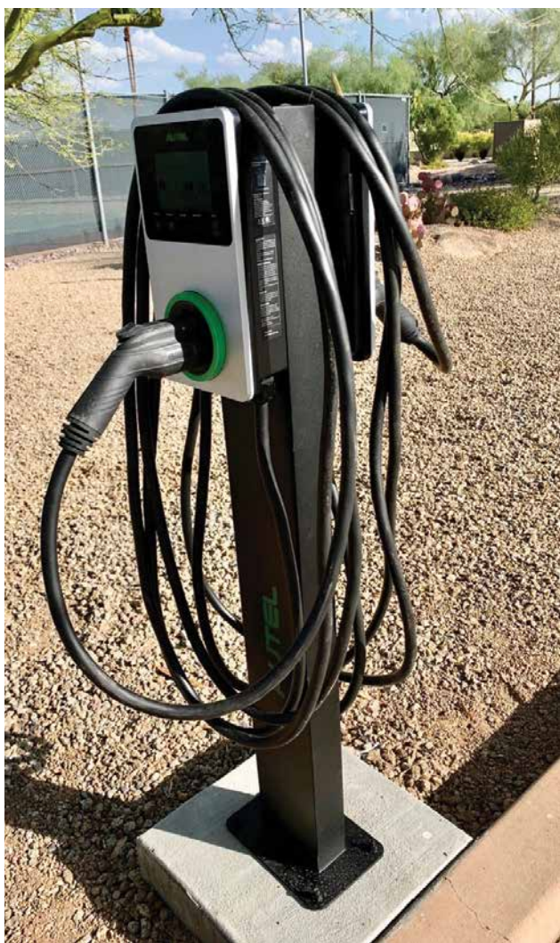
EV CHARGING SITE COMING TO RV
