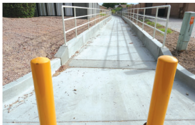
This drainage channel between Grande Boulevard and Rosita Drive was grant funded through the Flood Control District of Maricopa County. (Image courtesy of Town of Fountain Hills)
