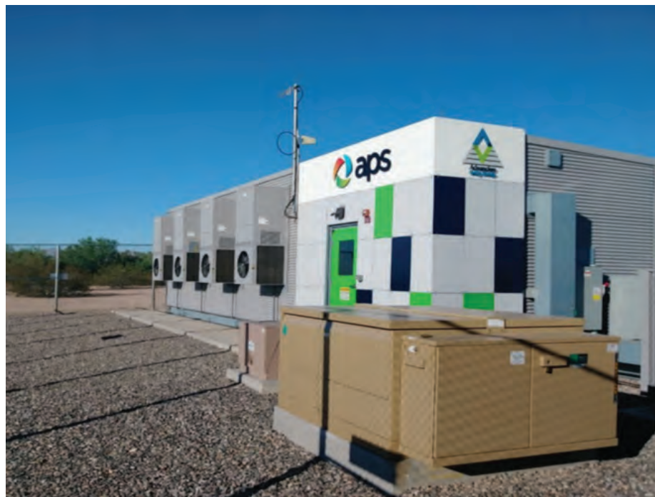
BESS units now have rules for how close they can be to homes in Surprise. (Courtesy city of Surprise)
